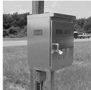
Permanent Automatic Traffic Recorder
