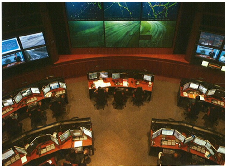
GDOT is using remote communications to actively manage traffic signals from the Transportation Management Center.
